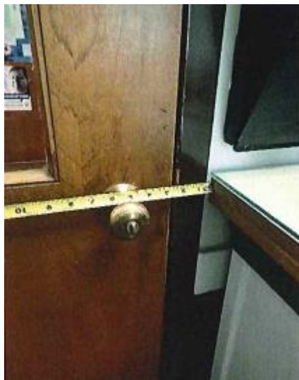
Figure 40: Non-compliant door hardware at Town Hall
