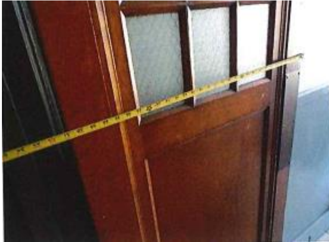
Figure 51: ADA non-compliant door width
