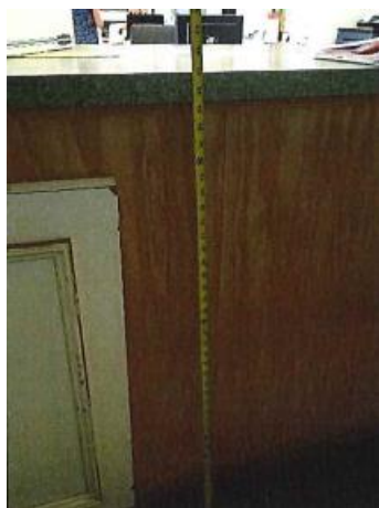
Figure 41: Non-compliant counter height
