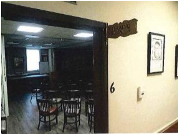
Figure 38: Non-compliant signage in Town Hall
